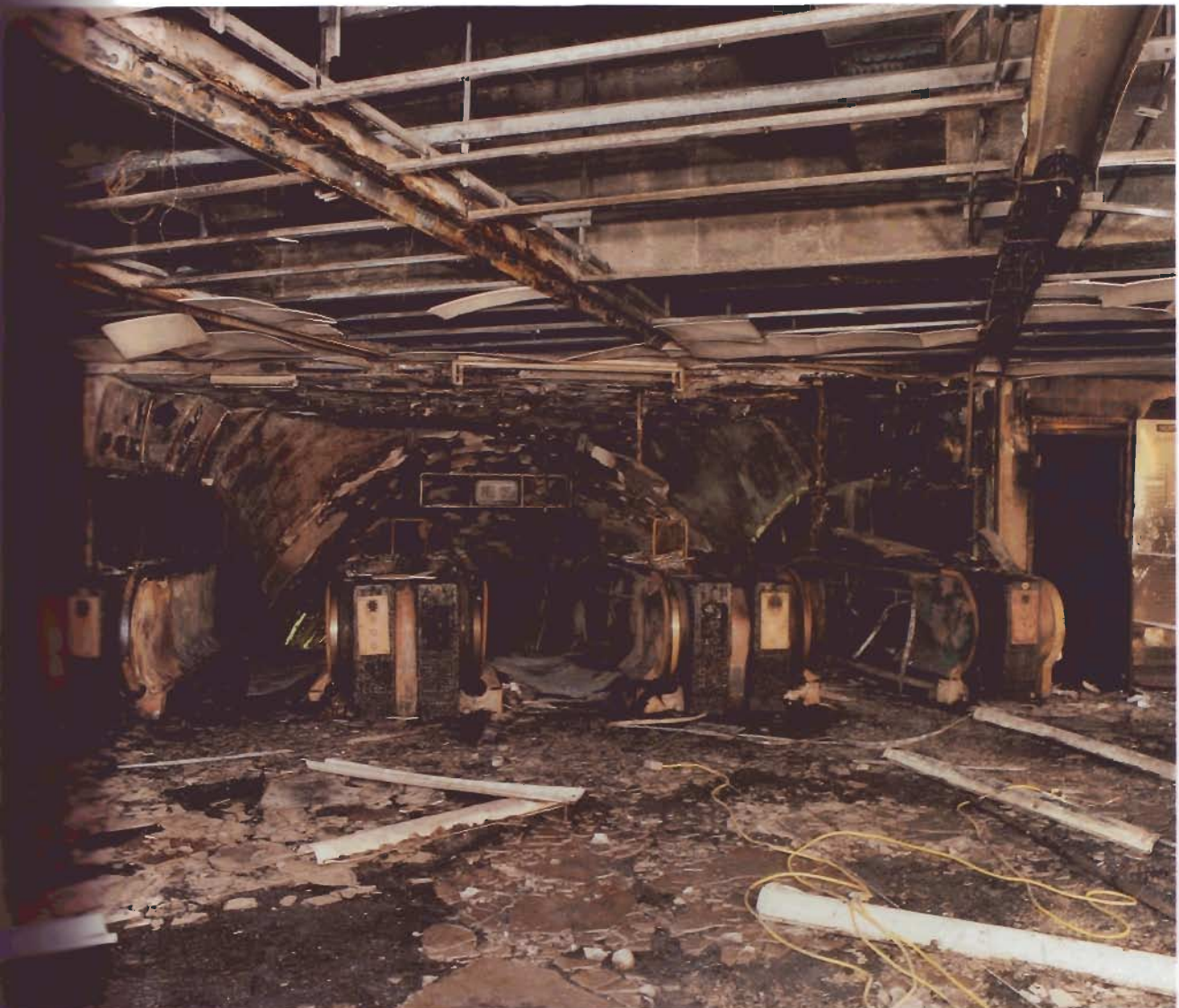
Top of the Piccadilly Line escalators seen from the ticket barriers showing fire damage
