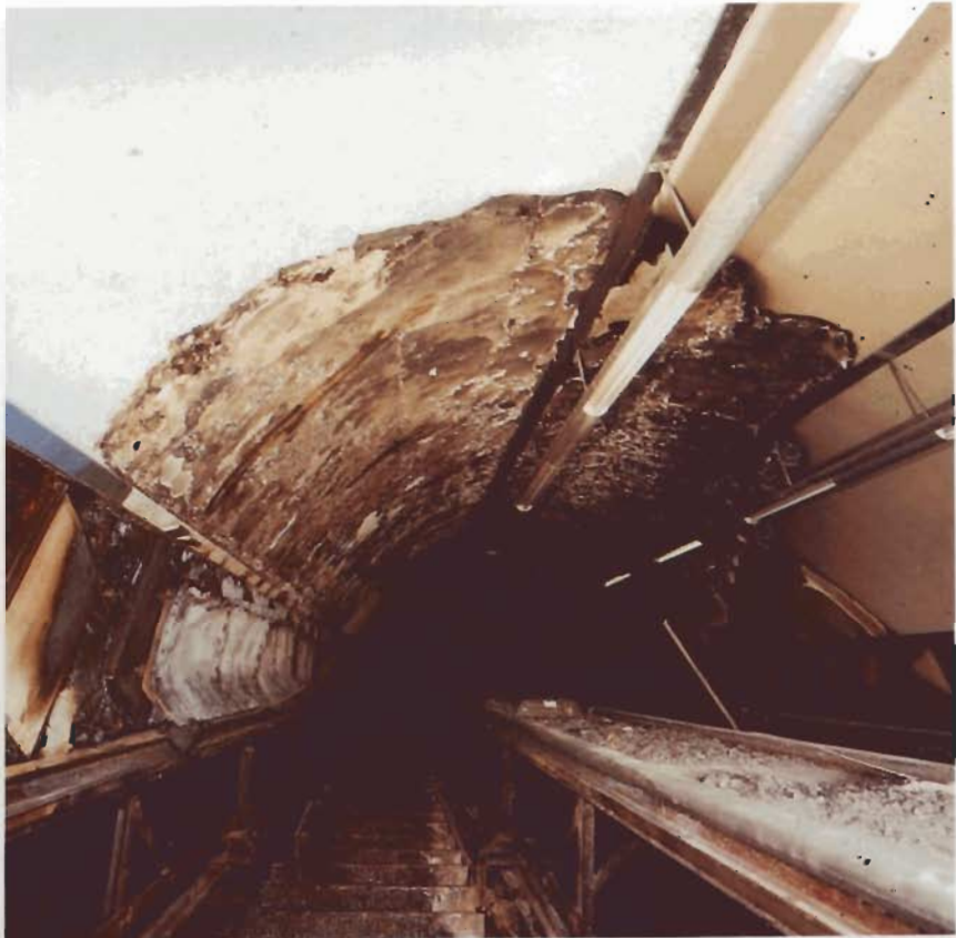
General view of fire damage in Piccadilly Line escalator shaft, looking up escalator 4 towards the tube lines ticket hall
