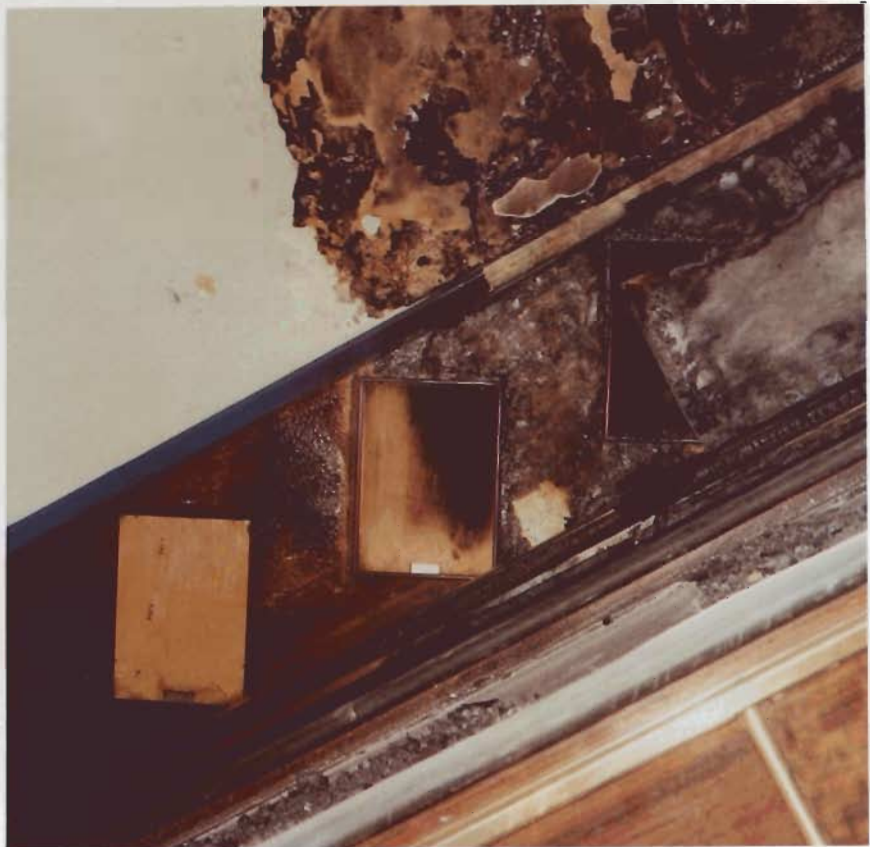
Damage to ceiling, fascia board and advertisement panel above escalator 4
